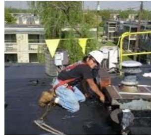
Good example of fall protection!
