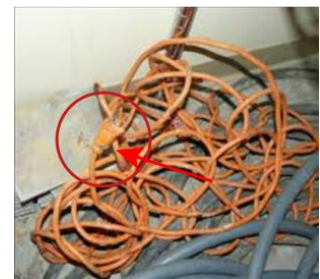
This cord was removed from service
