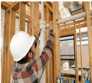
Contractor not wearing safety glasses
