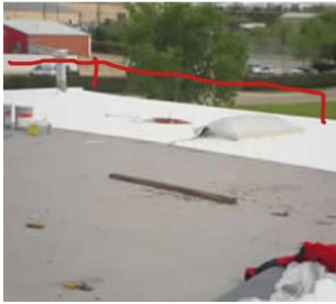
Need warning lines installed in area marked in red
