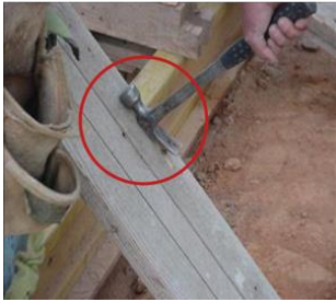
Nails were removed or bent down on several boards of scrap lumber
