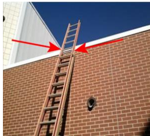
Ladder not secured
