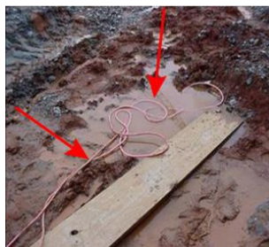
Flexible cord near job trailer should be relocated
