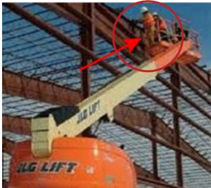
Observed one of the ironworkers standing on midrail when I arrived.
