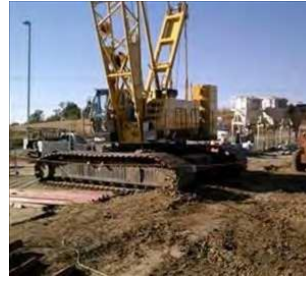
This crane has radius guard, but it should be flagged
